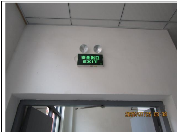
Exit sign and emergency light
