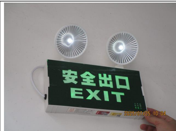
Emergency light test
