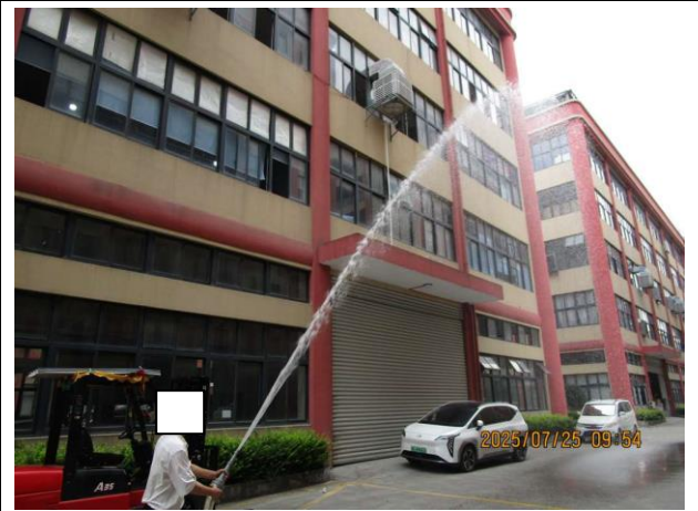
Fire hydrant test
